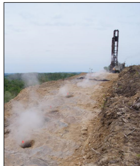
Fig. 8 Grout injection holes venting combustion gases at the Scotch Hill mine fire, Newburg, West Virginia, USA.
