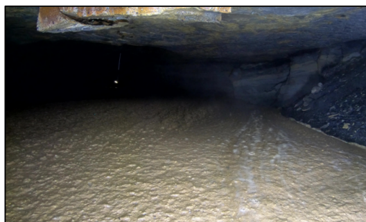
Fig. 11 Foam transported sand backfill being placed in a room and pillar coal mine.
